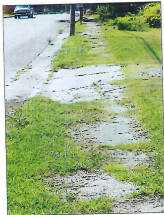
Bridgeton is already working to repair and replace many of the sidewalks that are in poor condition, like this one on B Street near Academy St.
